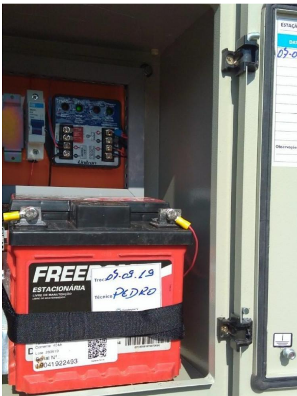
Foto 9 – Interior do Painel.
